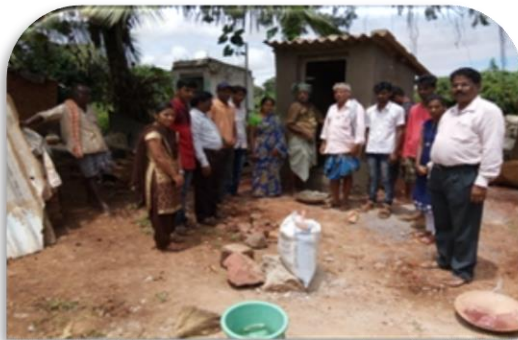
Toilet construction site visited by NSS Program Co-ordinator Dr. M. B. Dalapati.
